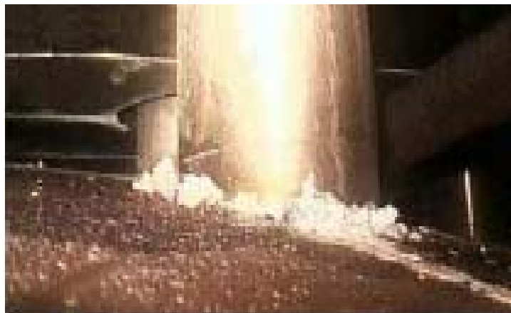
Figure 1 - Boric Acid Crystals Resulting from Primary Pressure Boundary Leakage (picture taken from lecture 13b)
